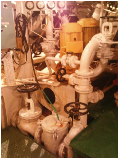
Picture 2.1.1.1 Lower floor of machine room
