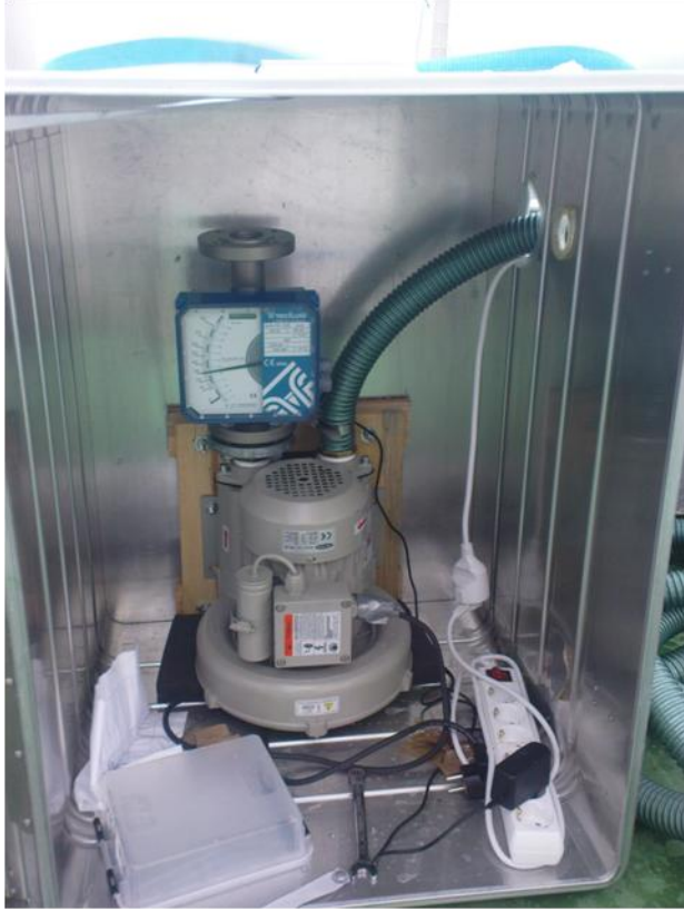
Picture 2.7.1 Pump and flow meter inside box.
