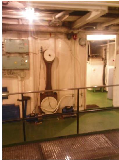
Picture 2.1.1.2 Impeller pumps, Kingston in background.
